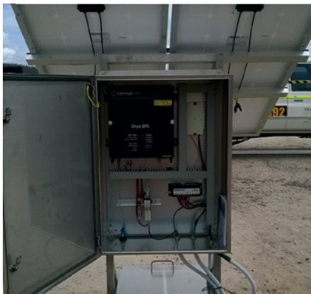
Oryx+ DTS unit installed onsite
