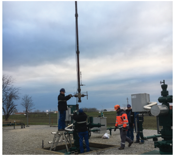
PulseEight ICV installation
